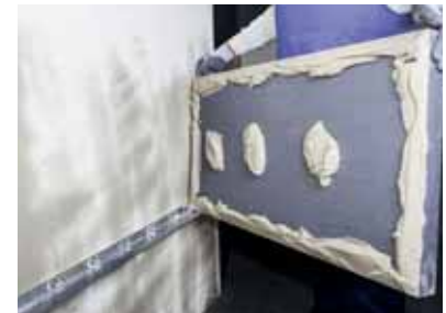
Figure 3 While applying adhesive mortar to the back of the insulation board, care is taken to prevent it from overflowing at the edges.
