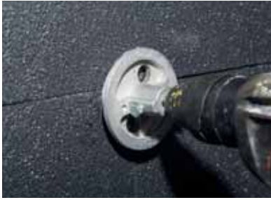
Figure 1 Counterboring by using apparatus is needed in order to place the wall plug head completely and to prevent thickness.
