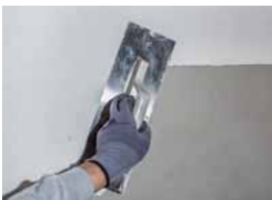
Figure 1 Teknosistem Mineral Textured Decorative Plaster is applied on the surface with trowel.
