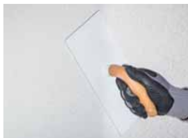
Figure 2 A plastic trowel is passed over the surface to form a texture before it dries.
