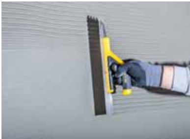
Figure 1 After adhering Teknosistem thermal insulation boards and applying wall plugs, two layers of surface plaster is applied. Teknosistem Plaster Mortar prepared is applied homogenously on the surface with a steel trowel.
