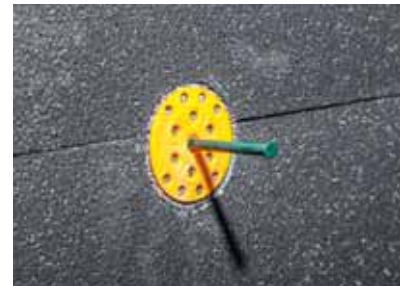
Figure 3 Wall plugs are placed in the holes, and nails are completely driven.
