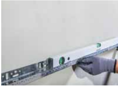
Figure 1 In the first step of the application; gaps, indentations, and protrusions between the wall and the Teknosistem Socle Profile are corrected using wedges of varying thicknesses, and the surface is measured with a surface level.
