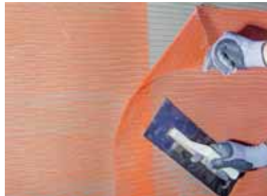
Figure 2 The glass-fiber mesh should be applied on the first layer of surface plaster when it is still wet by pressing from top to bottom and stretching widely, without folding, and placing at an equal distance from the insulation board to the whole surface. In joints, glass-fiber meshes should always be overlapped for 10 cm.
